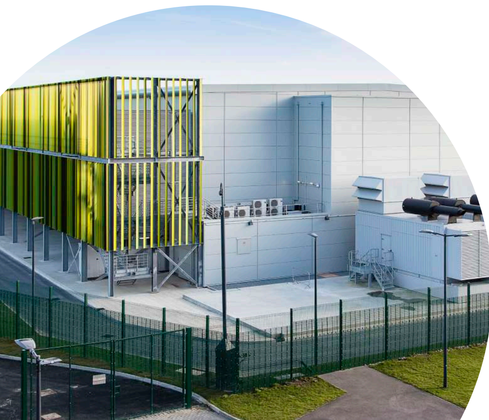
Kao Data's KOLON-01 data centre (Harlow) is home to the UK's fastest and most powerful supercomputer, NVIDIA's Cambridge-1. Picture Credit: Kao Data
